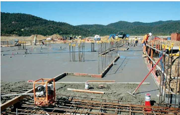
Port of Airlie's first ground floor suspended deck was poured on July 3.
